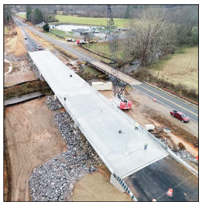
This substantially larger new bridge is replacing its 80-year-old counterpart on SR 66, which was deemed "structurally obsolete and functionally deficient" as far back as 2001. Photo/GDOT
